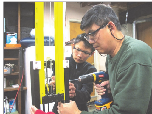
Miles Chan assists Mr. Xie in routing the electrical wires in the elevator.
